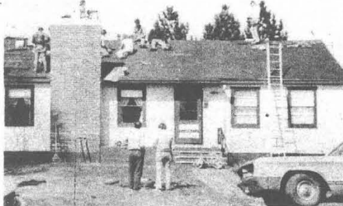
PATCHWORK — Duluth, Minn., members help repair the roof of the 27-year-old home of the Morkens April 27. (See "Church Activities," this page.)
