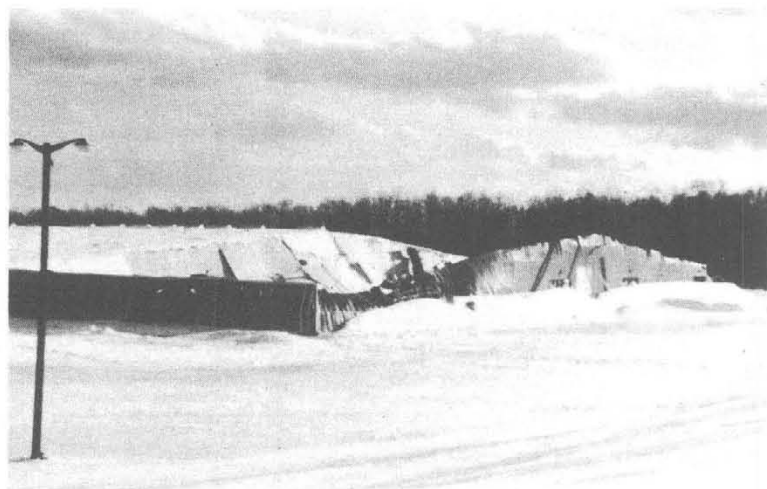
ROOF CAVES — The Feast building at Mount Pocono, Pa., suffered a disastrous cave-in Jan. 28 after snow and ice accumulated on its roof during a storm. The damage may mean no Feast at the Poconos in 1978. (See article, page 1.)
