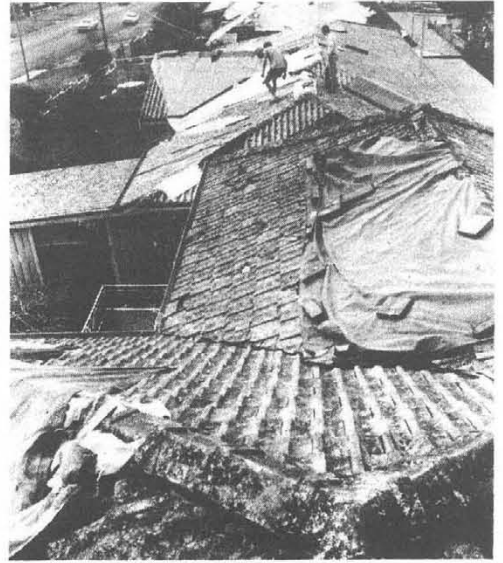
TOOWOOMBA HAIL — Residents of Toowoomba, Australia, cover their roofs with tarpaulins after a hailstorm that caused nearly $10 million in damage Jan. 10. (Photo courtesy Toowoomba Chronicle)
