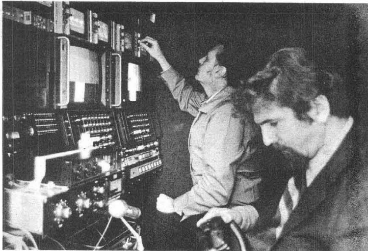
INTERIOR CONSTRUCTION — Lee Pettijohn, left, adjusts camera controls and Bob Wickersham installs audio equipment during the video pod's construction.
