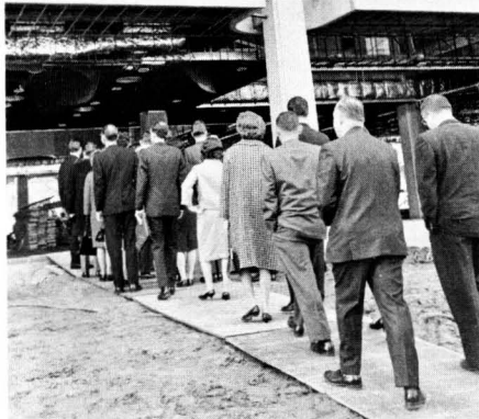
CONSTRUCTION PROGRESS —Touring ministers enter Dining Hall to view progress of building.
