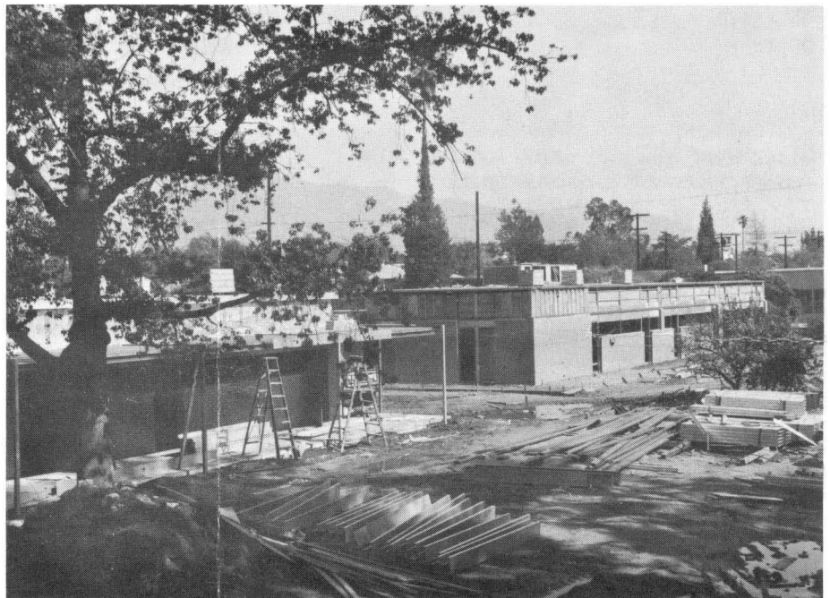
NEW SCHOOL—Rheem Manufacturing Company has construction well advanced for new grade school building. Made of modular components primarily for speed, cost approximates stucco-plaster.
